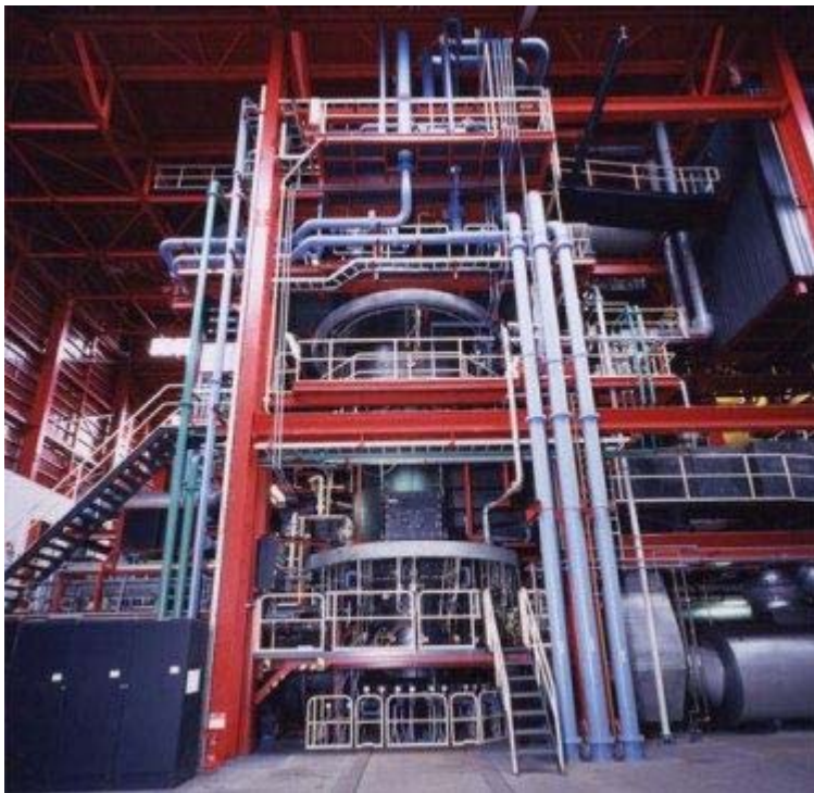
(High-temperature pyrolysis chamber. Image credit: Interstate Waste Technologies)
